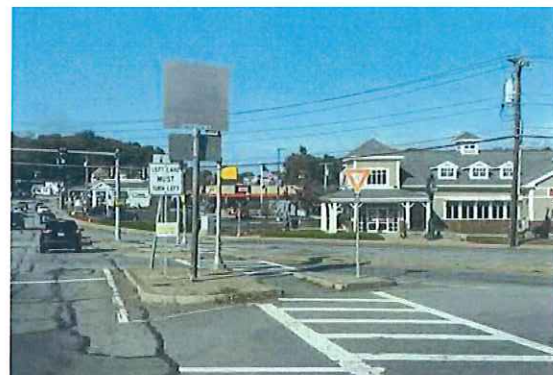
Pictured: Crosswalk across right-turn slip lane from Cambridge Street northbound to Winn Street where no pedestrian signal indications or pushbuttons exists.
